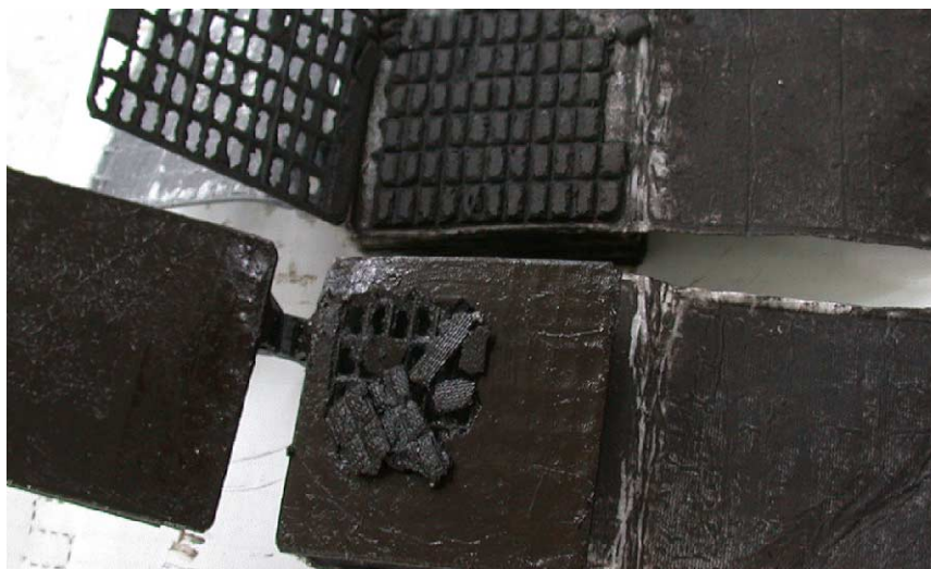
Fig. 5. Condition of positive plates from failed battery.
